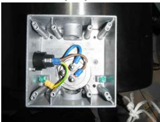
Internal view showing wiring to 2400w element:
