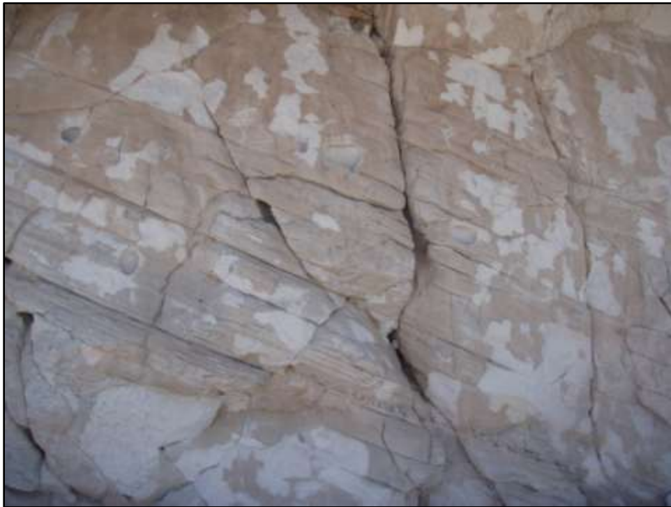
48J01241, Feature 1, fire damaged rock art panel. Close up of panel showing inscriptions and fire damage. Taken by Ardeth Hahn, 7/14/2010.
