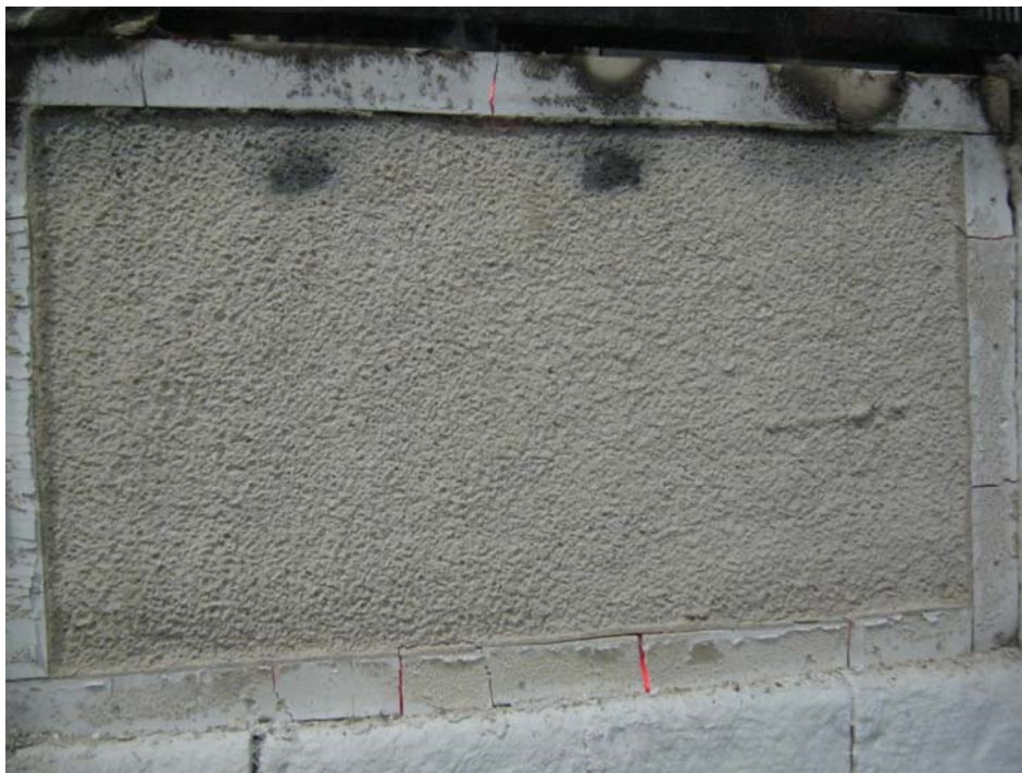
Test #2 - Exposed Side After the Fire Test
