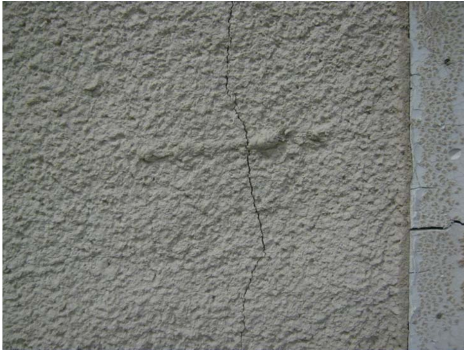
Test #2 - Exposed Side After the Fire Test (note: crack extends through the surface and cement backer board)
