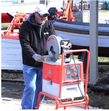
Scott Chandler at work trimming the pavers to fit. Scott has been the mastermind behind this project!
