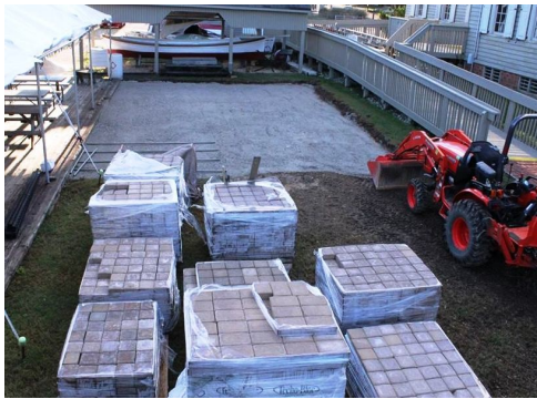
Scott and his team have excavated the area to be paved, and filled and leveled the gravel bed. Now for the hard part—installing the pavers!
