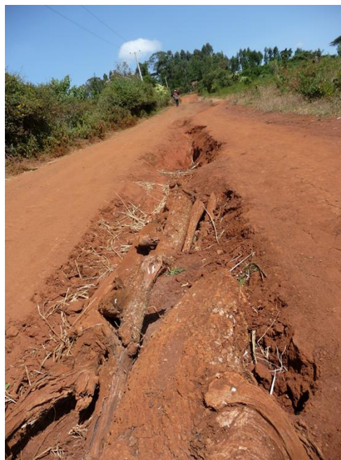
Fig 11: Road erosion in Mua Hills.
