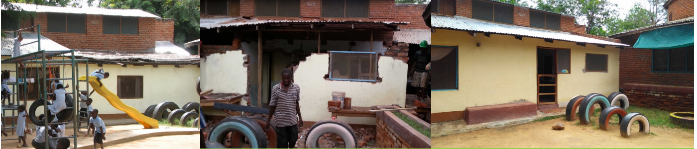
So-- This became .....this..... became .....new admin offices .. Thank you for allowing it to happen!!
