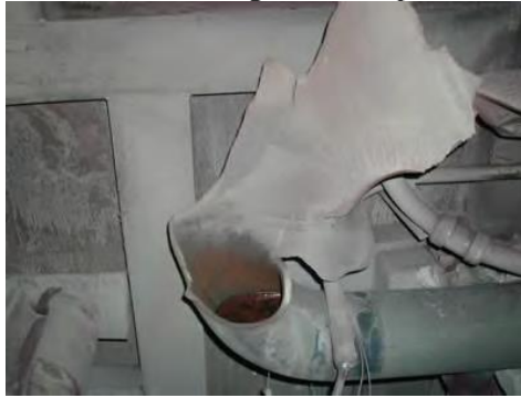
Figure 3: Hamaoka, Japan, Nuclear Power Plant, Piping Explosion, 6" Dia., Sch. 40 Pipe (Leishear [8])
