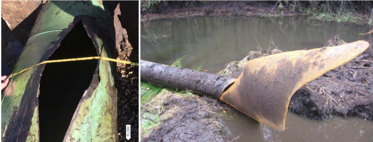
Figure 4: Typical Gas Pipeline Explosions Caused by Fluid Transients
