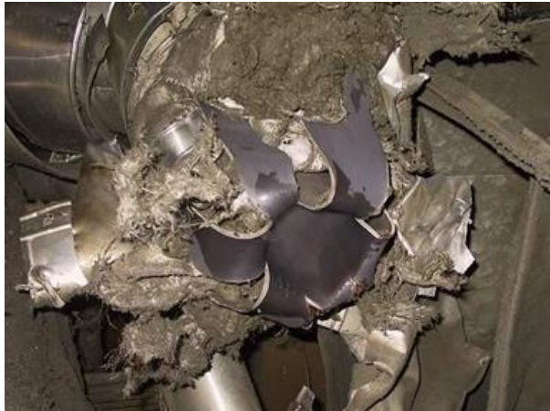
Figure 8: A Nuclear Power Plant Pipe Explosion Caused by Fluid Transients, Brunsbüttel
