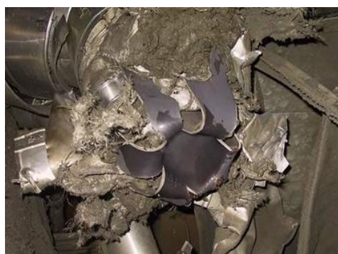
Brunsbuttel Piping Explosion
