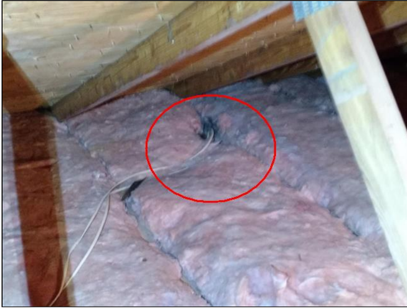
7.8 Item 16 (Picture) Light under there?
