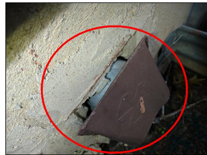
15.4 Item 3 (Picture) Old dryer vent under deck appears to be not in use. The foundation penetration should be sealed
