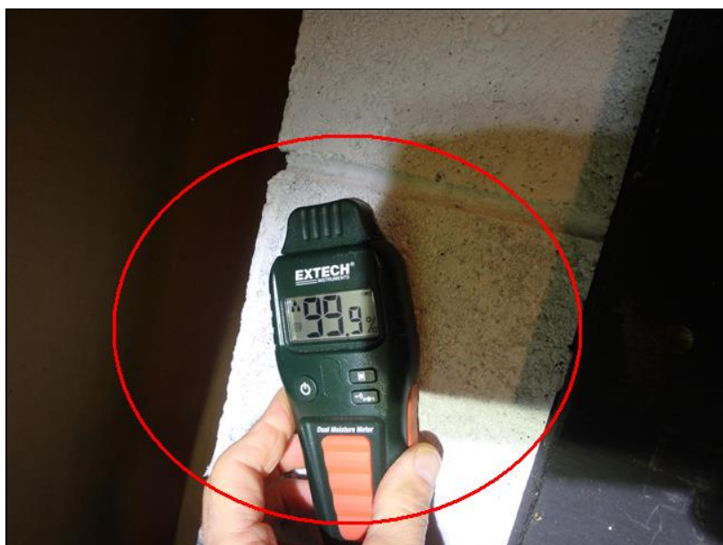
4.0 Item 10 (Picture) 99% moisture content on some of the foundation walls
