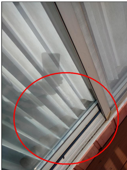
12.7 Item 1 (Picture) Failed window seals
