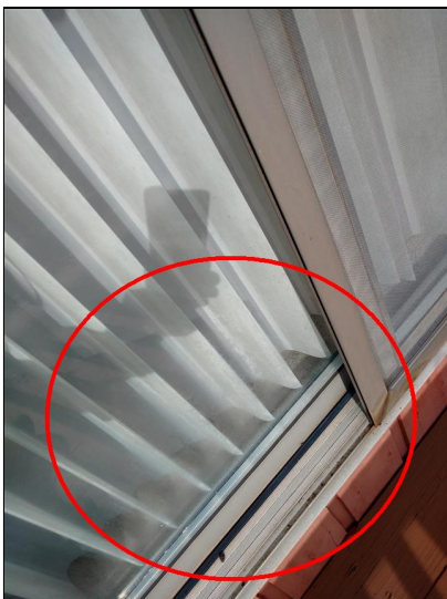
12.7 Item 1 (Picture) Failed window seals
