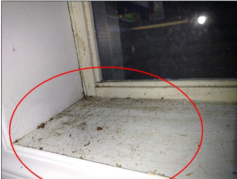
12.2 Item 11 (Picture) Moisture damaged basement window which doesn't open
