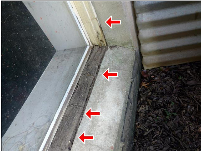
2.0 Item 14 (Picture) Basement window frame deteriorated
