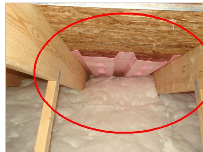
6.3 Item 2 (Picture) Example of venting
