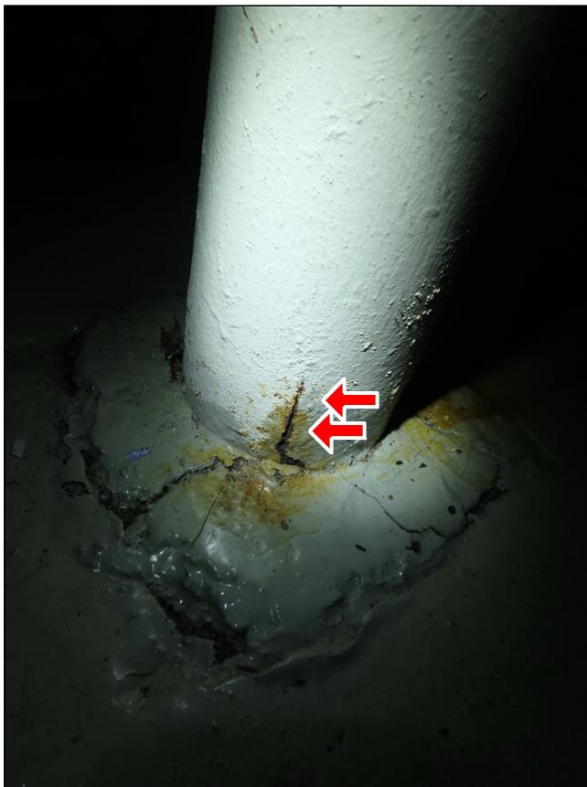
4.1 Item 4 (Picture) Cracked
