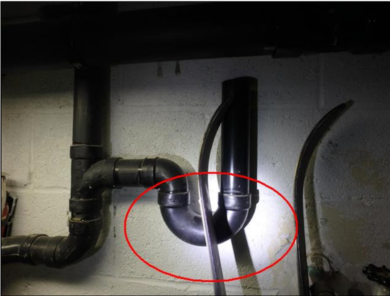
8.2 Item 2 (Picture) P-trap is probably dry/no water in it
