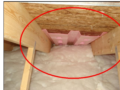
6.3 Item 2 (Picture) Example of venting
