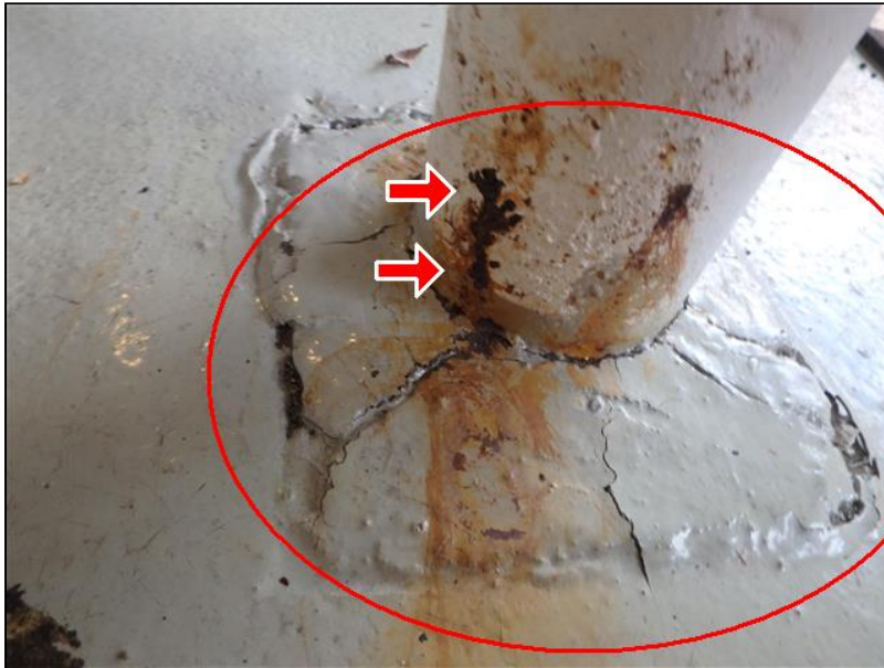
4.1 Item 2 (Picture) Cracked
