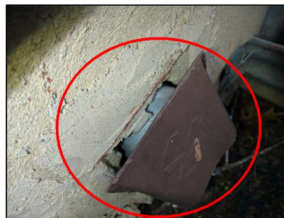
15.4 Item 3 (Picture) Old dryer vent under deck appears to be not in use. The foundation penetration should be sealed
