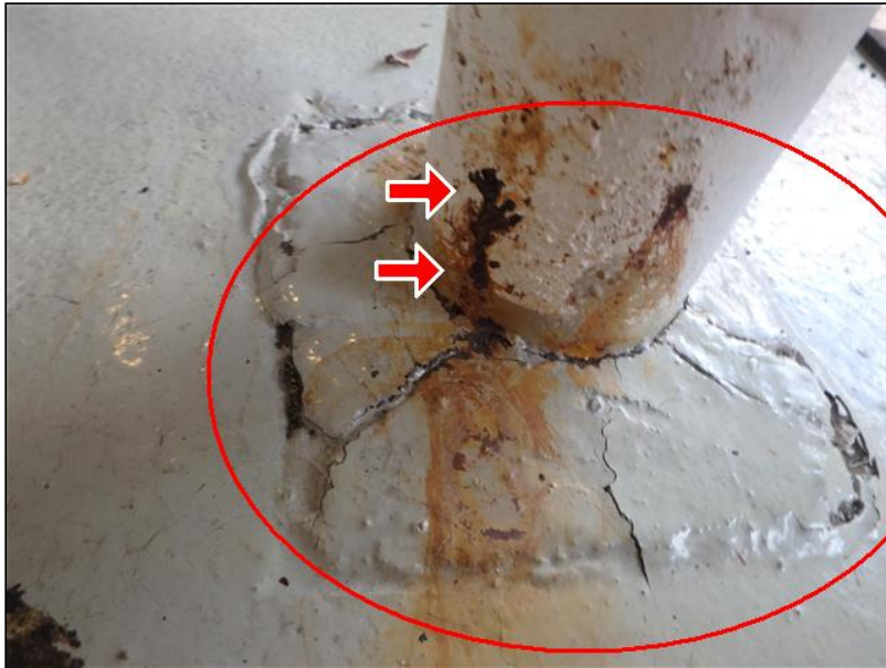
4.1 Item 2 (Picture) Cracked
