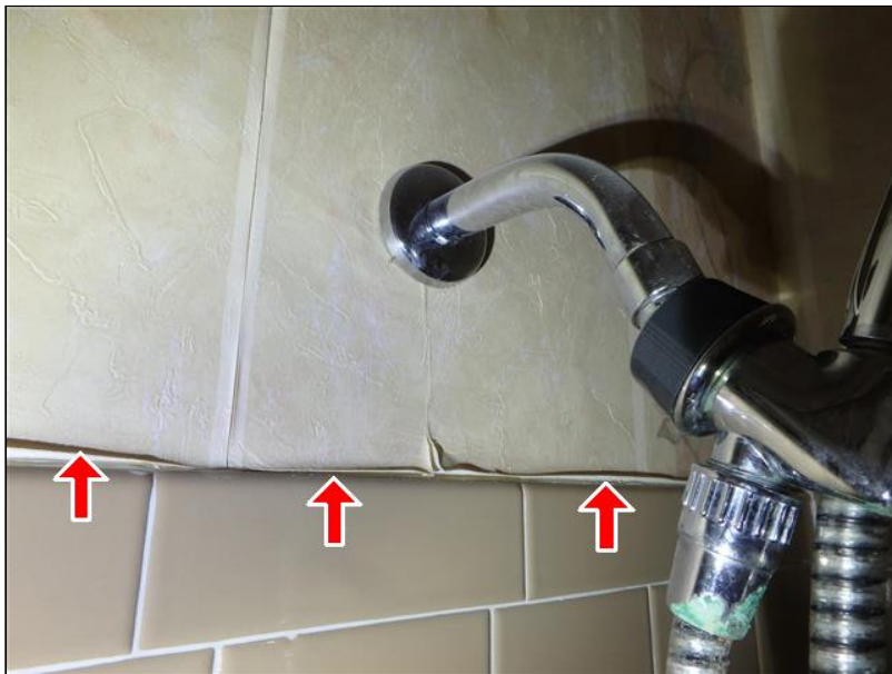
12.2 Item 4 (Picture) Wallpaper should not be in a shower area
