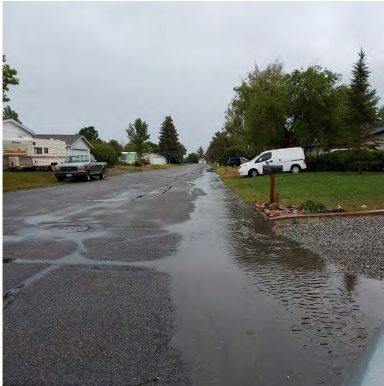
Photo 3: Flooding Along South Side of Buffalo Road
