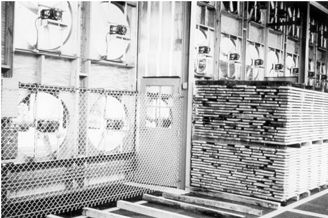
Figure 3—Fan shed air dryer draws air through the stickered packages of lumber.
