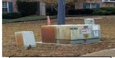
Rusted Utility Box
