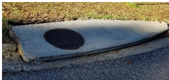
Broken Drainage Cover
