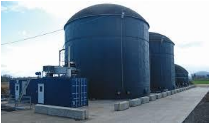
Manure Anaerobic Digester
