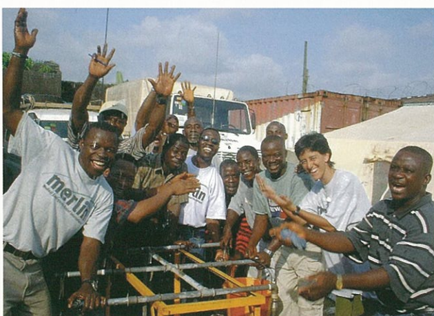
Water from the taps! Workshop participants celebrate completing an emergency water supply at the end of the Monrovia training.
