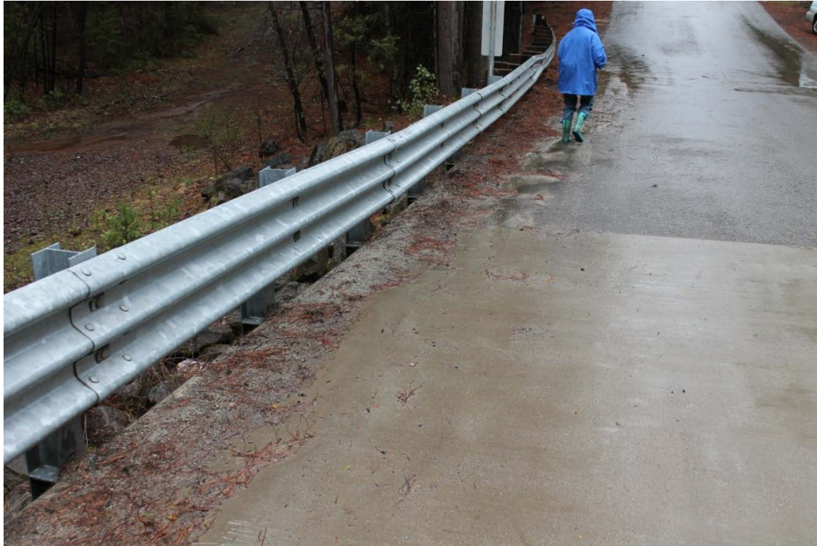
Figure 27: Sediment source on paved road leading to Rock Creek.
