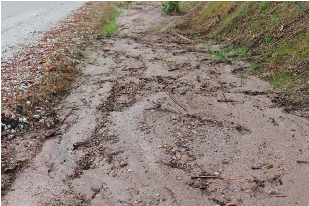
Figure 26: Sediment in roadside ditch in the Canyon Creek drainage.
