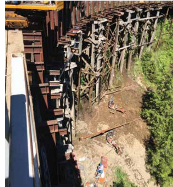
PHOTO 8 The flume is elevated by more than 12m (40ft) in some areas.
