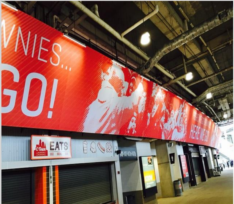
Cleveland Browns Stadium 310' by 13' Vinyl Banner mounted on steel structure with graphic fixed on the side.
