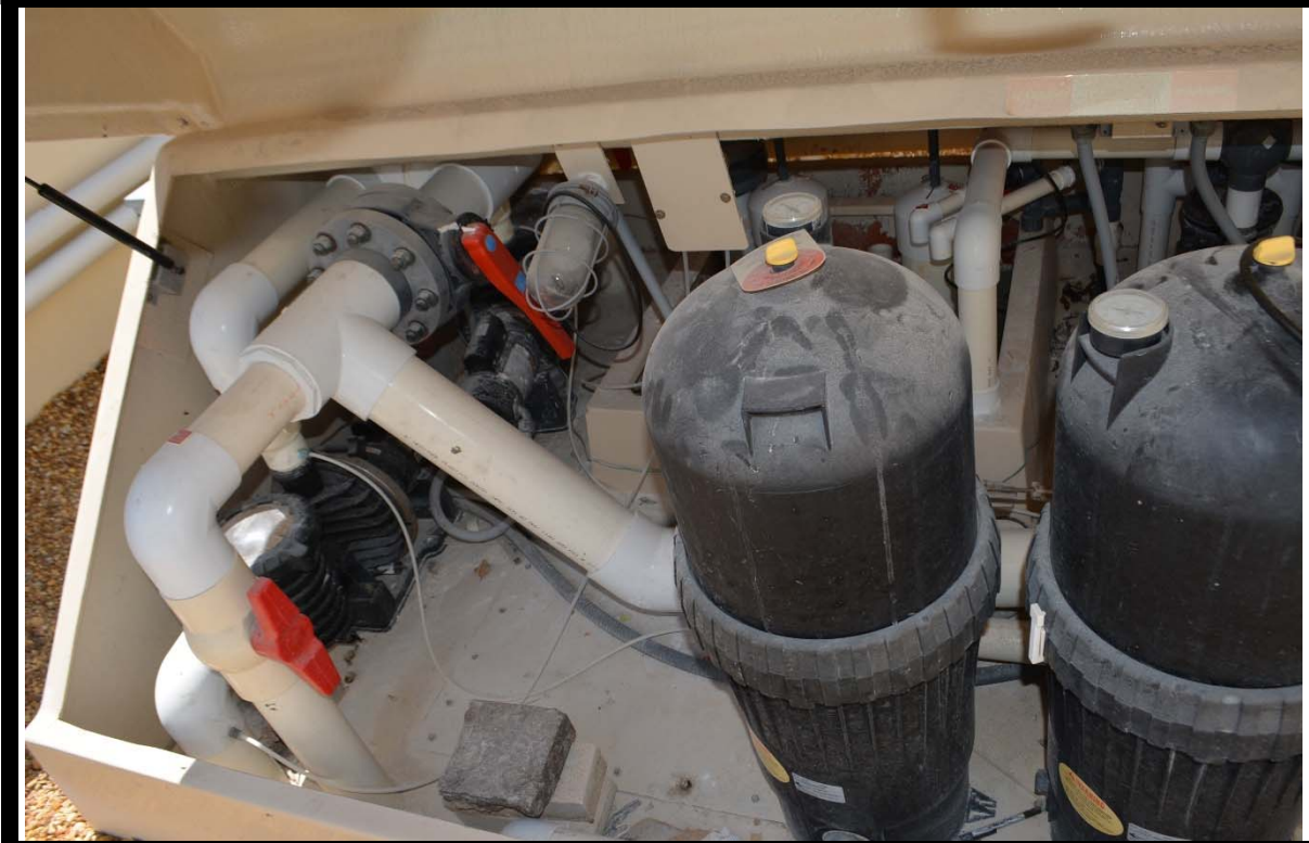
VIEW OF SWIMMING POOL EQUIPMENT
