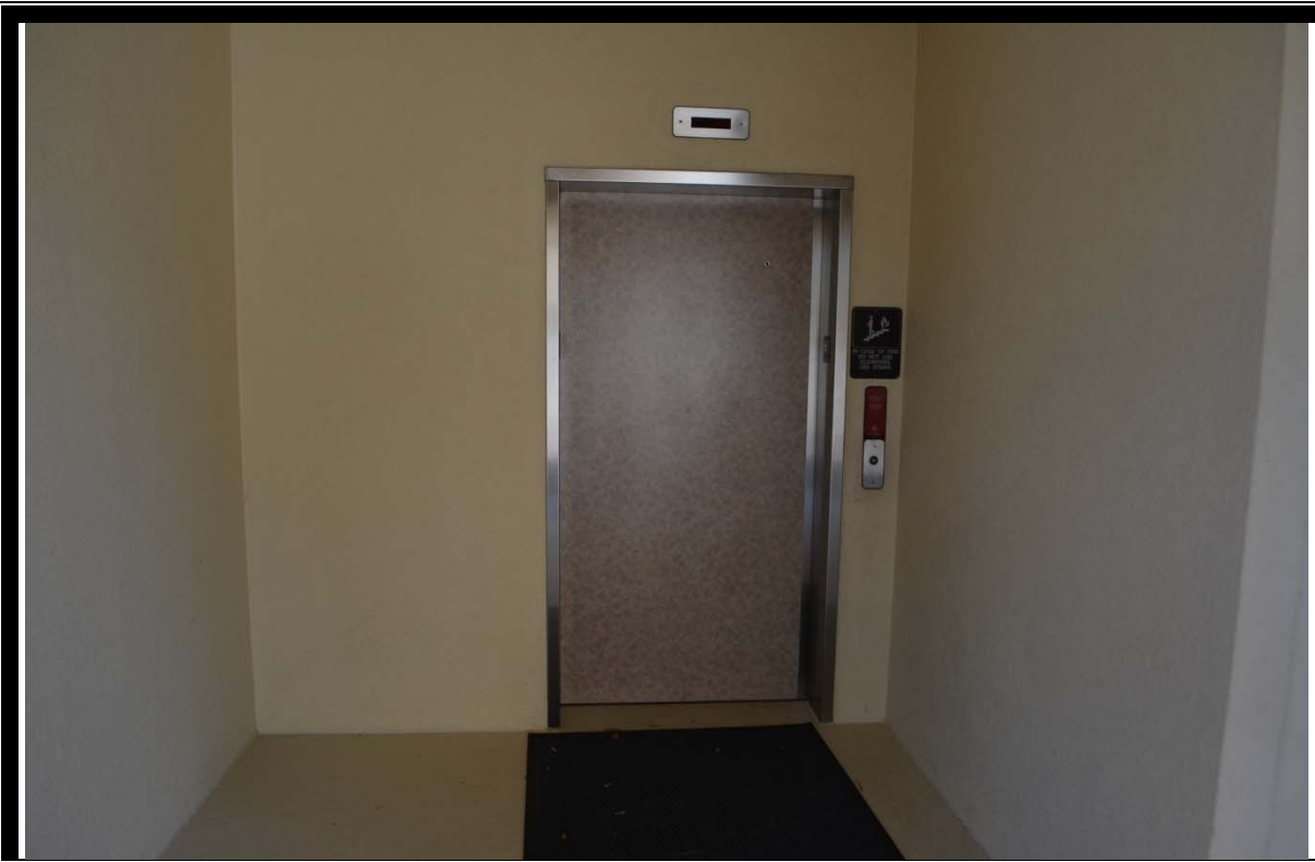
VIEW OF TYPICAL RESIDENTIAL BUILDING EQUIPMENT
