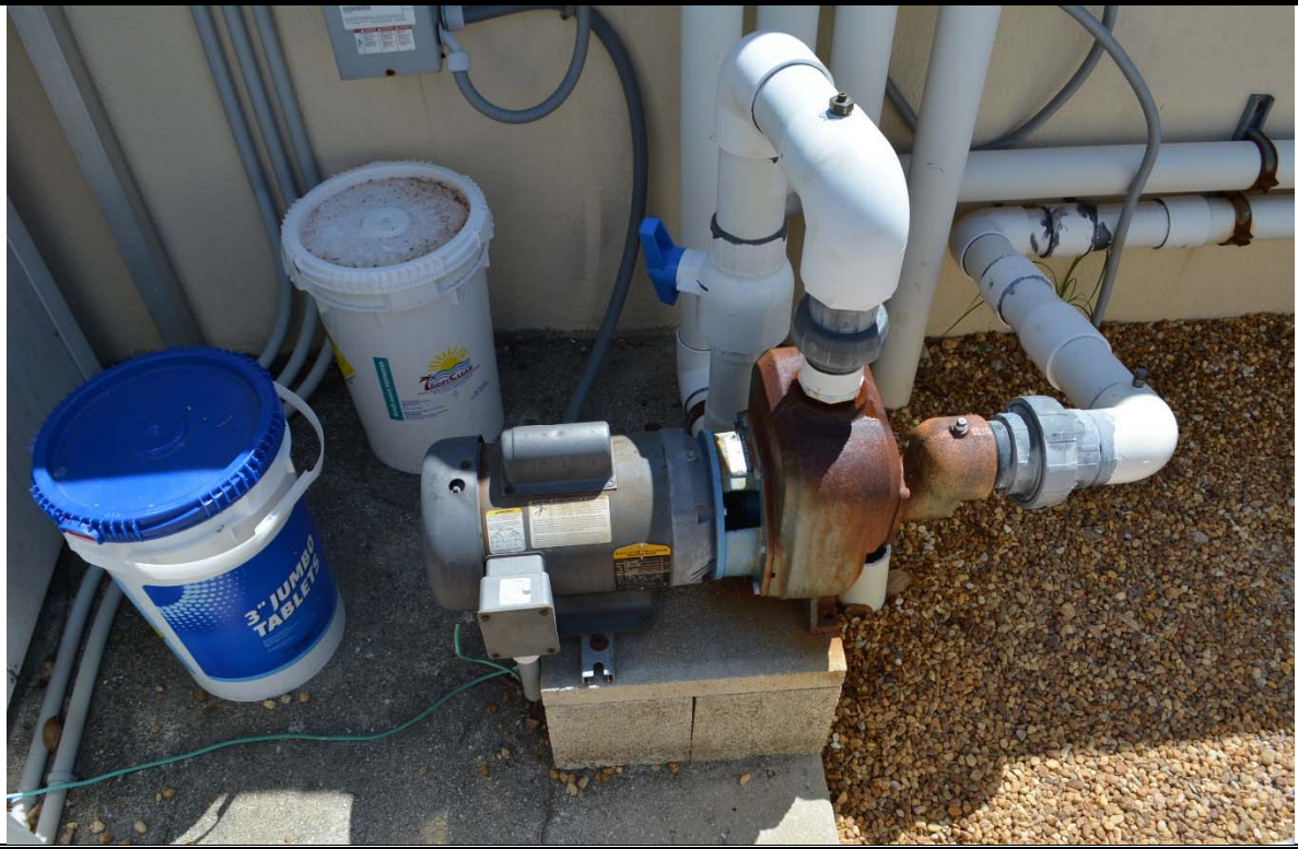
VIEW OF SWIMMING POOL EQUIPMENT
