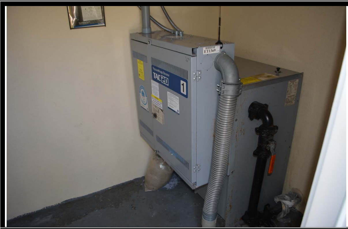
VIEW OF TYPICAL RESIDENTIAL BUILDING EQUIPMENT
