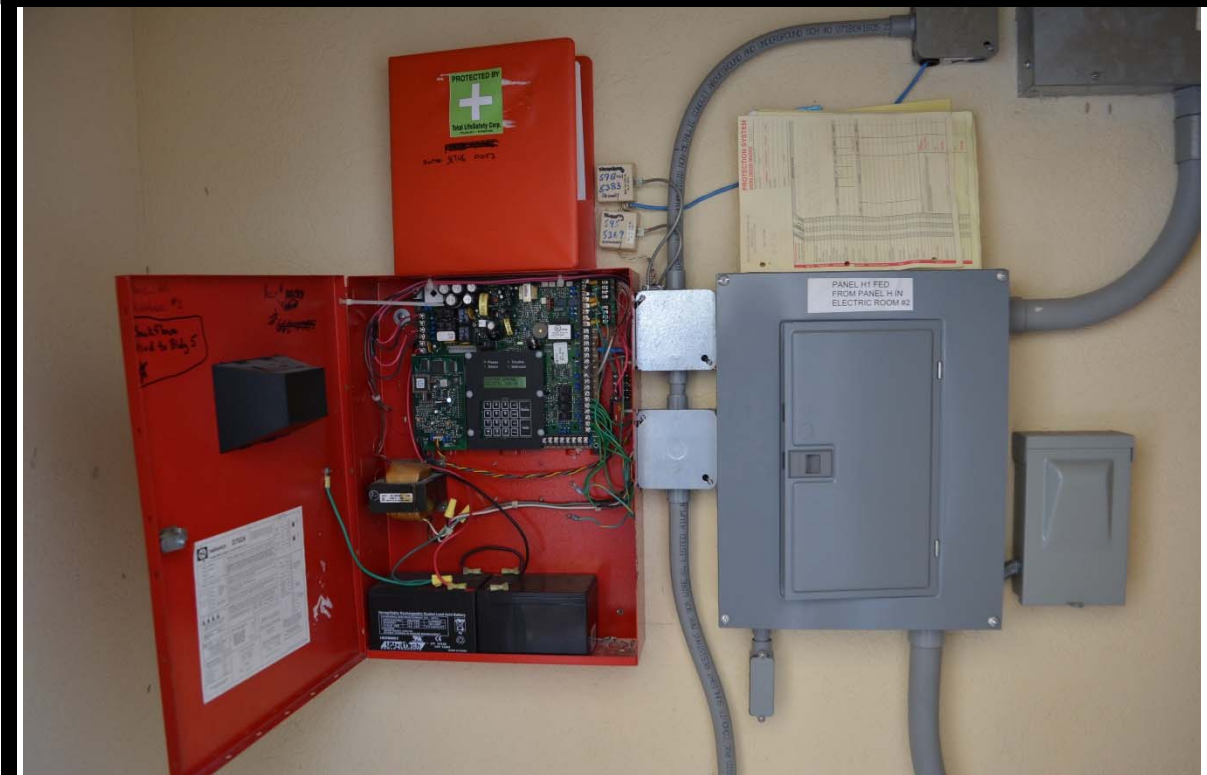
VIEW OF TYPICAL RESIDENTIAL BUILDING EQUIPMENT
