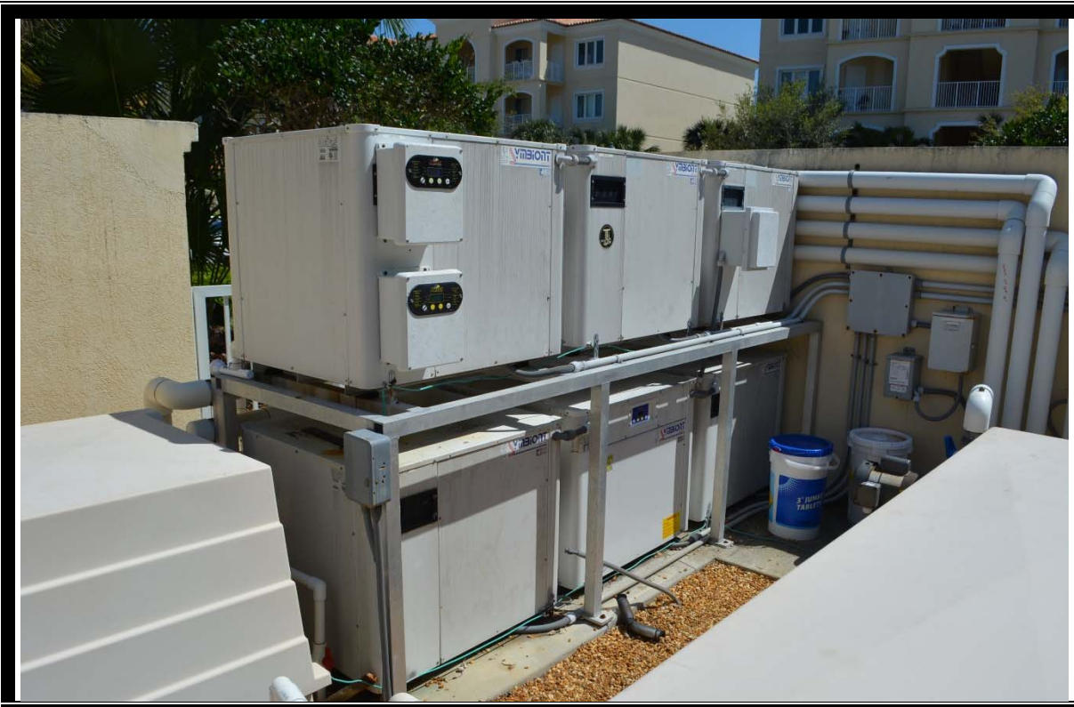
VIEW OF SWIMMING POOL EQUIPMENT
