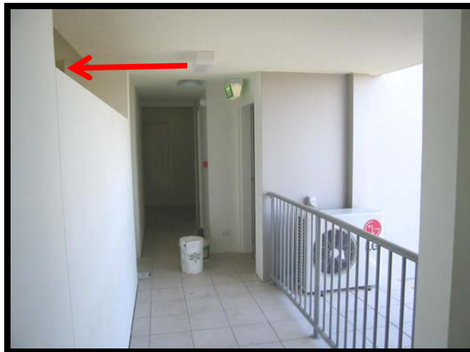
Figure 3 – Open Balcony – Opening to Unit shown at left.
