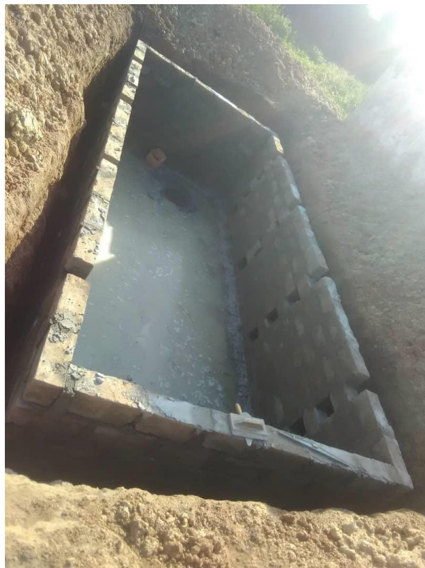
Fig. 32- Pit filled with water by rain.
