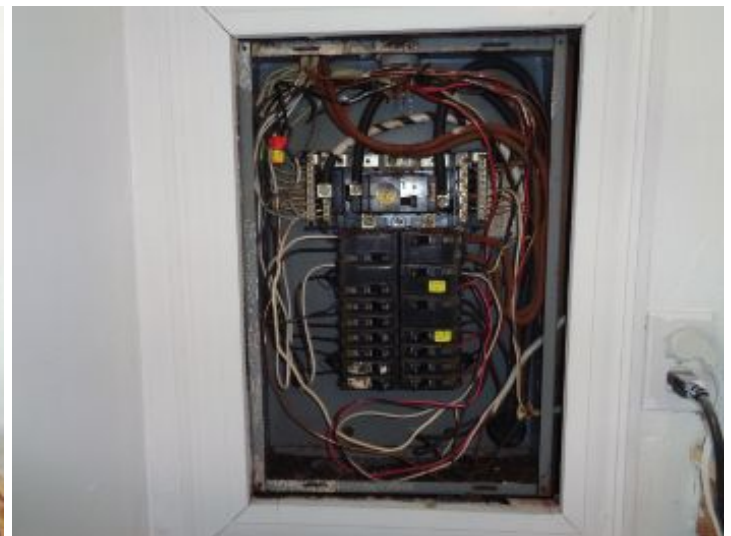
Electric, Heat, Water Heater Electrical Panel
