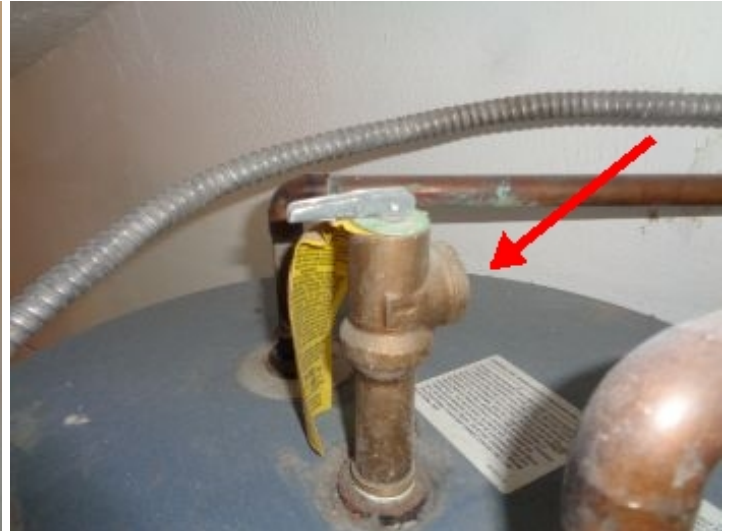
Missing Drain Pipe
