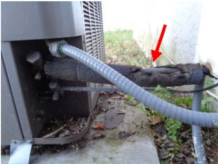
A/C unit pipe insulation
