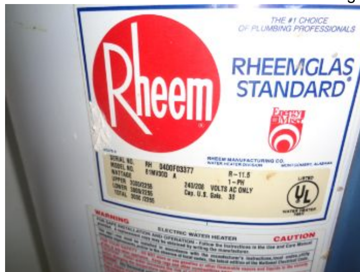
Water Heater Sticker Plate
