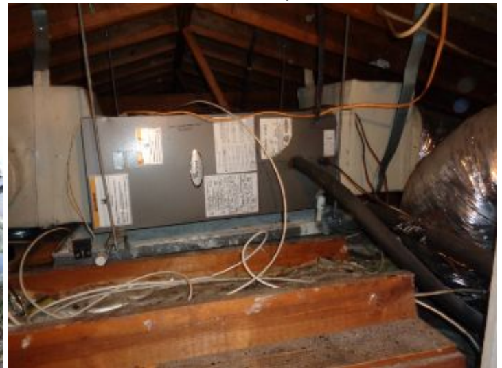
Electric, Heat, Water Heater HVAC Unit
