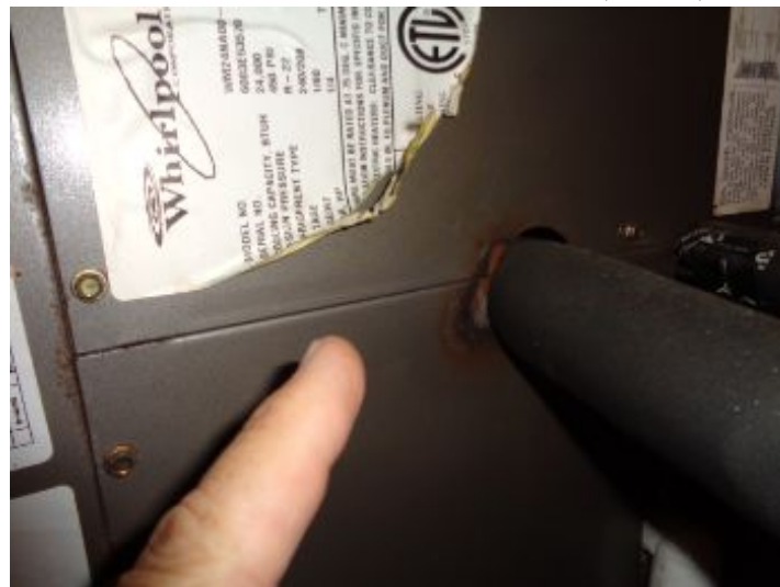
HVAC exterior burning
