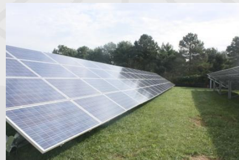
83kW Ridgely's Wastewater Treatment Facility, MD
