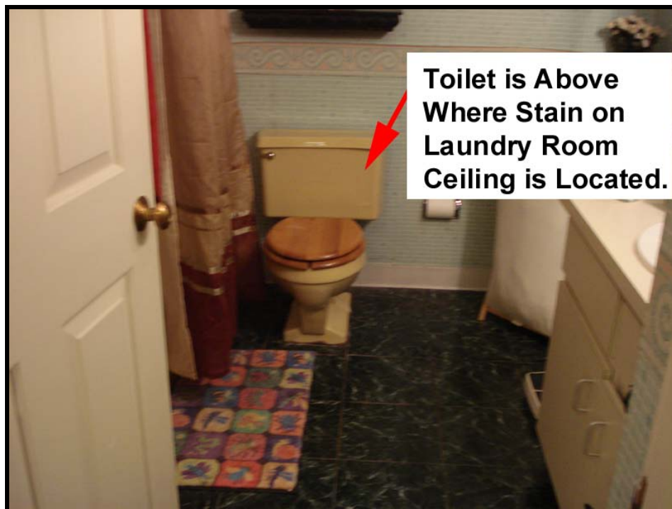
Up Stairs Bathroom Above Laundry Room – Image 7
