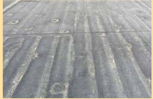
Example of rutting in polyisocyanurate insulation in an adhered EPDM membrane roof system
