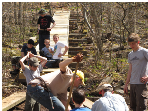
A new 200 foot board walk from the Searing site to the dam making the area more accessible for nature hikes at Winnebago.
