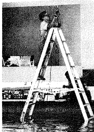
Photo courtesy of Corps of Engineers Electrical Construction.
