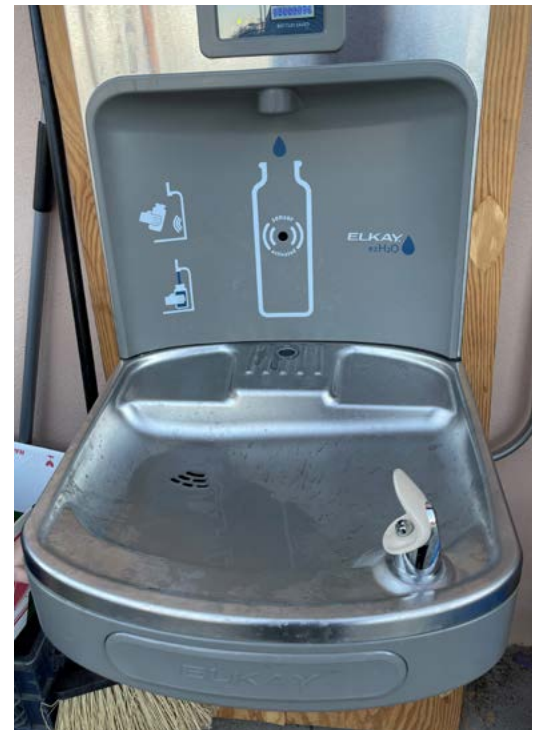
Above: Our water filling station
