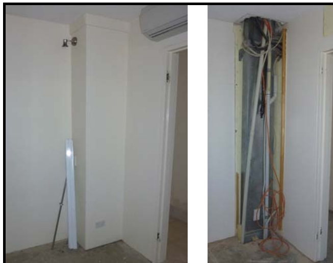
Figure 7 - From the same project. On the left in a bedroom showing an innocuous corner feature. On the right showing the bathroom exhaust duct with no dampers, openings up into the bedroom on the floor above and in to the bedroom lobby on the right. No fire stopping of penetrations.
