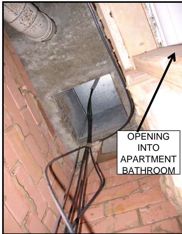
Figure 9 – From another project showing how the bathroom exhaust and services were accommodated in a masonry duct. This is looking upwards from the top floor through to the roof where the exhaust fan was located. An opening covered with a mirror mounted on plywood protected the opening to the bathroom! A grille through the brick wall to the bathroom served as the required ventilation.
