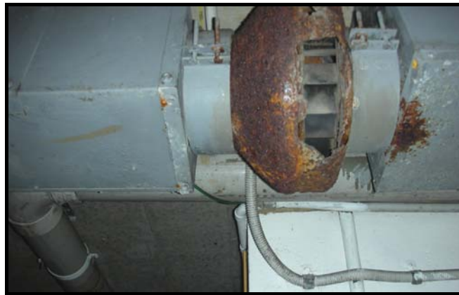
Figure 6 – Bathroom exhaust fan located in basement car park for the gymnasium in the same area. The makeup air was through a grille opening into the basement car park!
