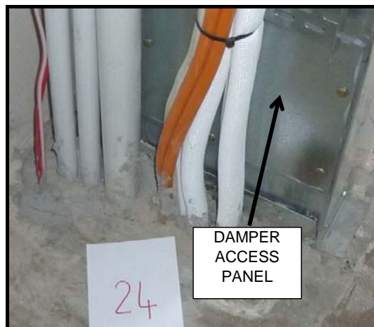
Figure 8 – again from the same project and after refurbishment. It shows the bathroom exhaust duct with its access panel for the damper and the surrounding penetration acceptably fire stopped.
