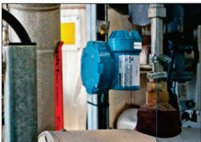
Figure 5 – Acoustic monitors mounted next to steam traps took less than ten minutes per trap, and the system paid for itself in energy savings within a year
