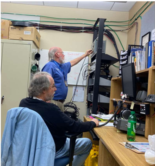
Preparing EOC radio room for practice drill.
