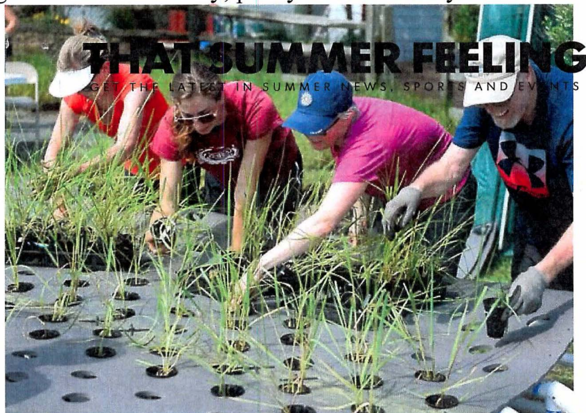
One-hundred and thirty floating treatment wetlands will be placed along bulkheads in many of South Bethany's canals to help treat stormwater runoff from up to 345 acres of surrounding land on Tuesday, June 19, 2018. (Photo: Staff Photo by Megan Raymond)
