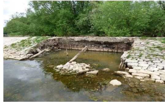
Fig. 2: Partial collapse of the weir wall (©Keith Walton, 2020)
