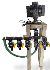
Sump Recovery Pump
