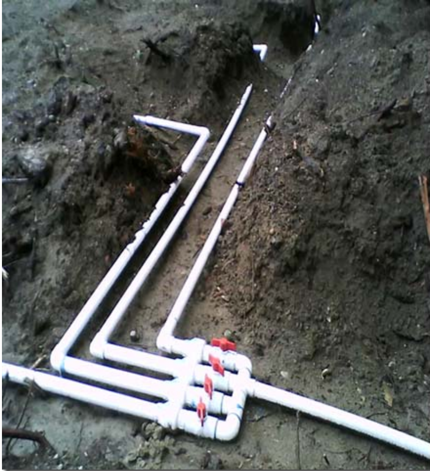
Manifold with four lateral connections. The valves control the amount of effluent to each lateral. Each valve is adjusted differently depending on the elevation of each lateral.
