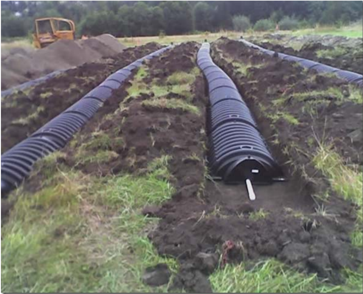
Drain field with four lateral trenches on a sloping site. Each individual trench is level from end to end. Although each trench is on a different elevation.
