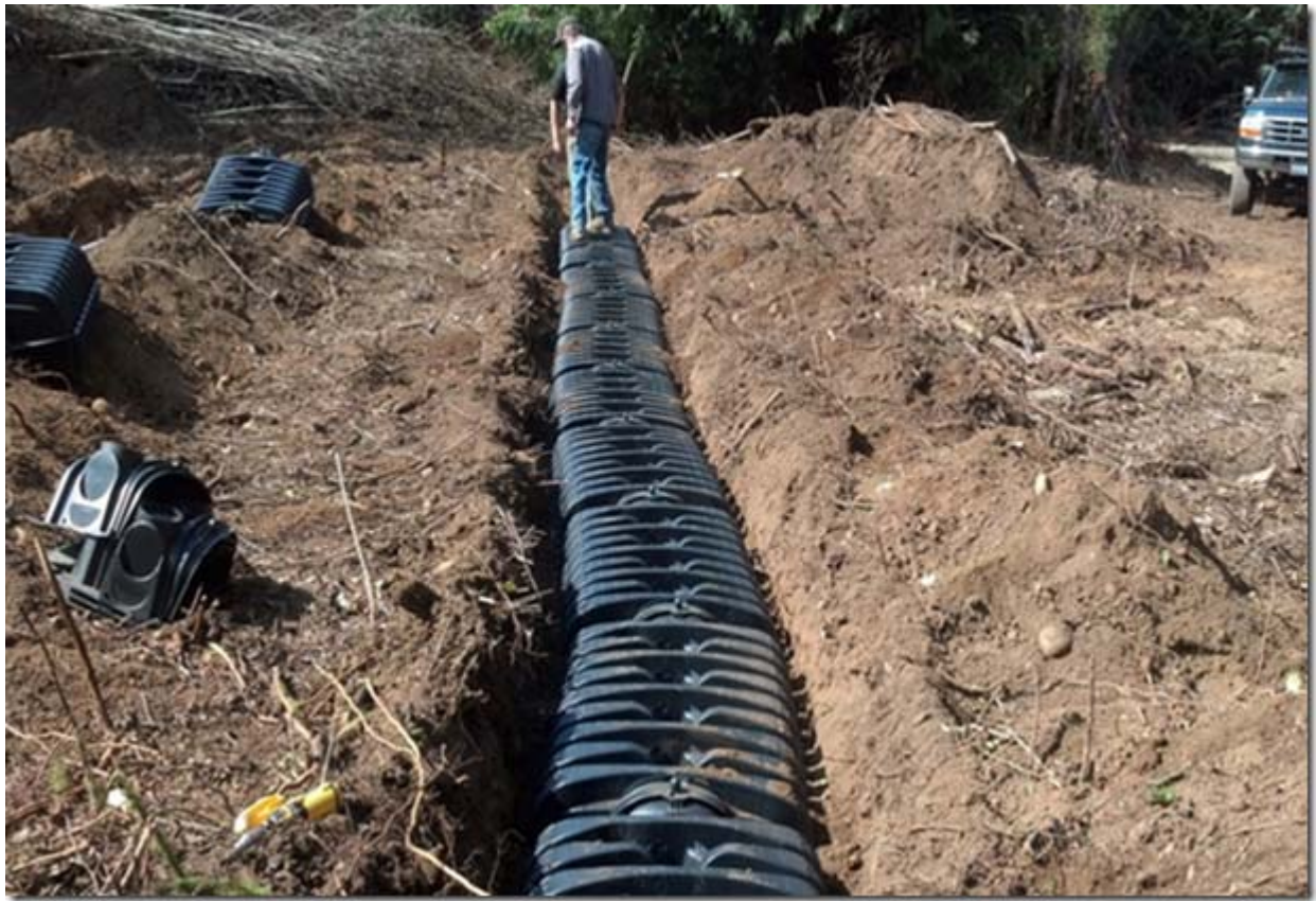
This was heavily timbered prior to clearing. We used low-profile chambers to minimize the overall trench depth.
