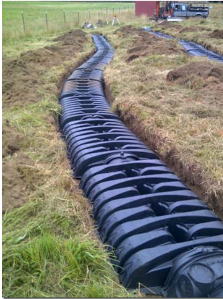
Low profile chambers on sloping site. Notice how the trenches follow the contour of the site to maintain equal depth over the entire length of the lateral.
