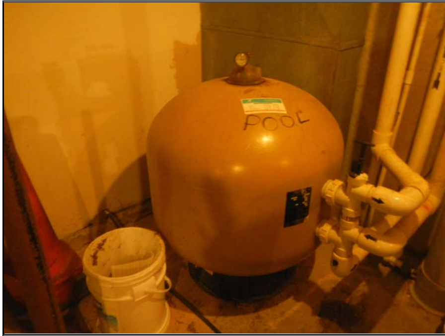
Photograph 7: Typical view of pool filter
