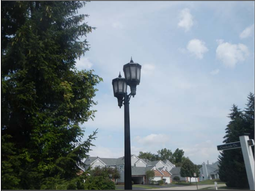
Photograph 13: Typical view of pole light fixture
