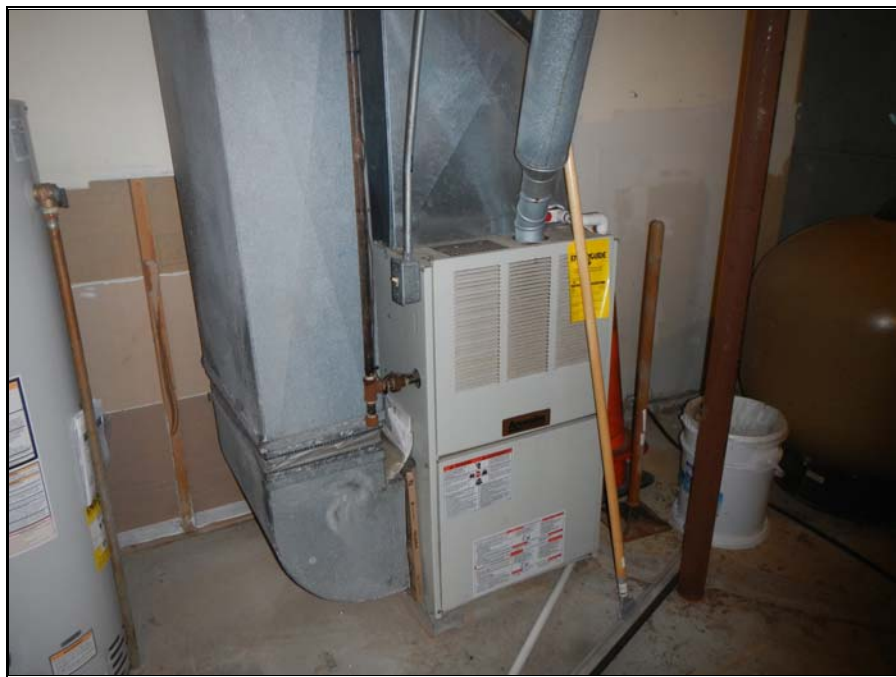
Photograph 4: Typical view of clubhouse forced-air furnace
