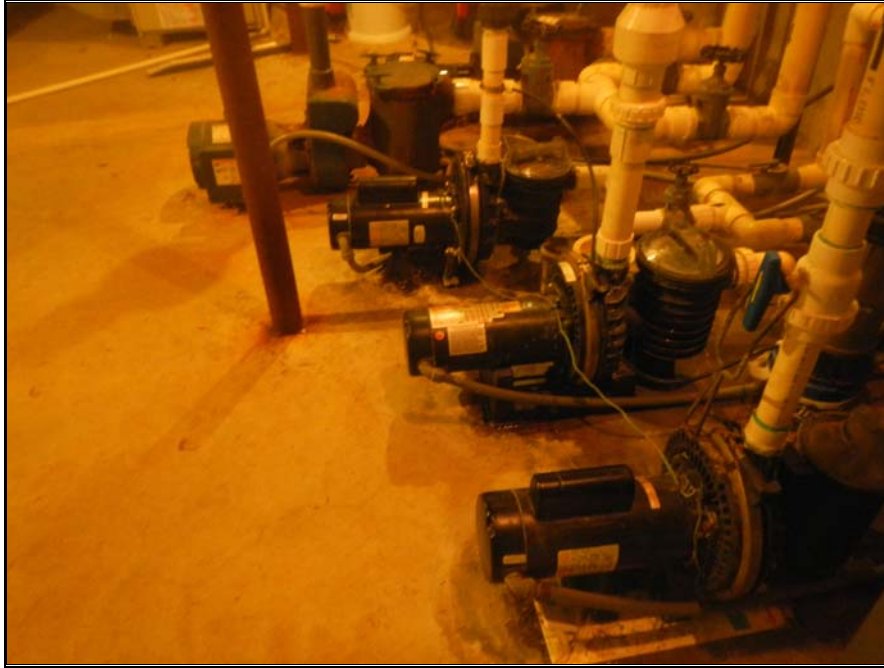
Photograph 5: Typical view of pool/spa pumps
