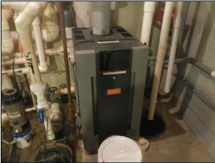
Photograph 6: Typical view of pool heater
