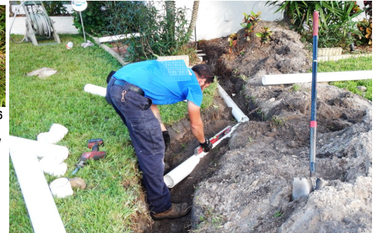
PVC pipe installation. Correct slope is critical & is being checked with a level
