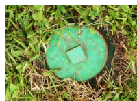
Close-up view of the existing 6 inch clean out, approx 25 ft out from the house. If the City Public Works Dept ever responds for a sewer blockage (on their side) at your home, they will install one of these if one doesn't already exist.
