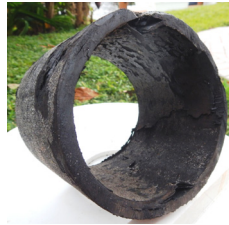
Piece of the old Orangeburg pipe, 4 inches inside diameter
