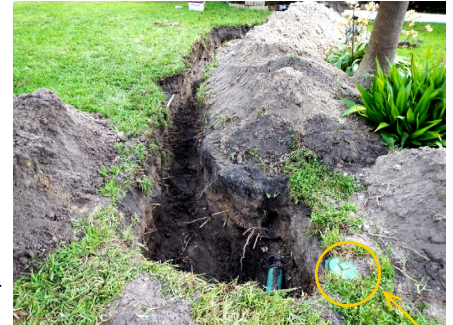
The trench is finished from the house to the 6 inch city cleanout
