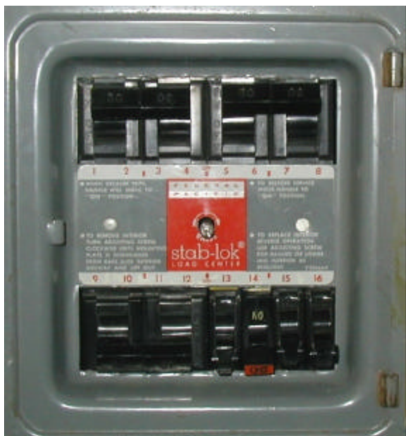
Figure 2 – Breakers that are on when down
