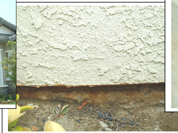
Corroded Weep Screed due to soil contact and sprinkler spray.
