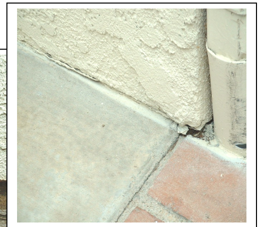
Weep Screed inappropriately covered with concrete flatwork.
