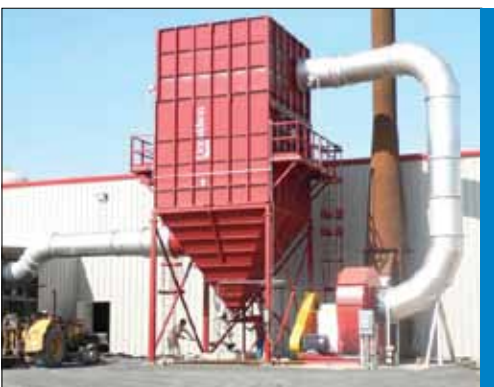
324MBWS10 at a glass manufacturing facility
