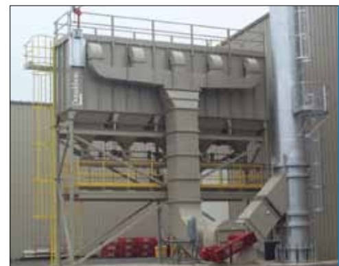
405MBT8 at a brick manufacturing facility
