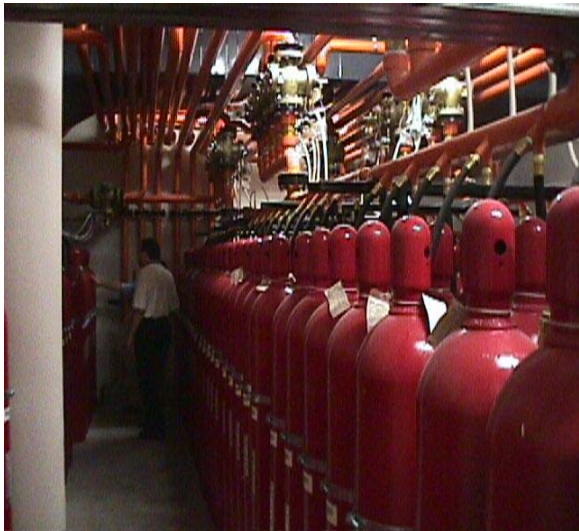
CO 2 SYSTEM CYLINDER BANK
