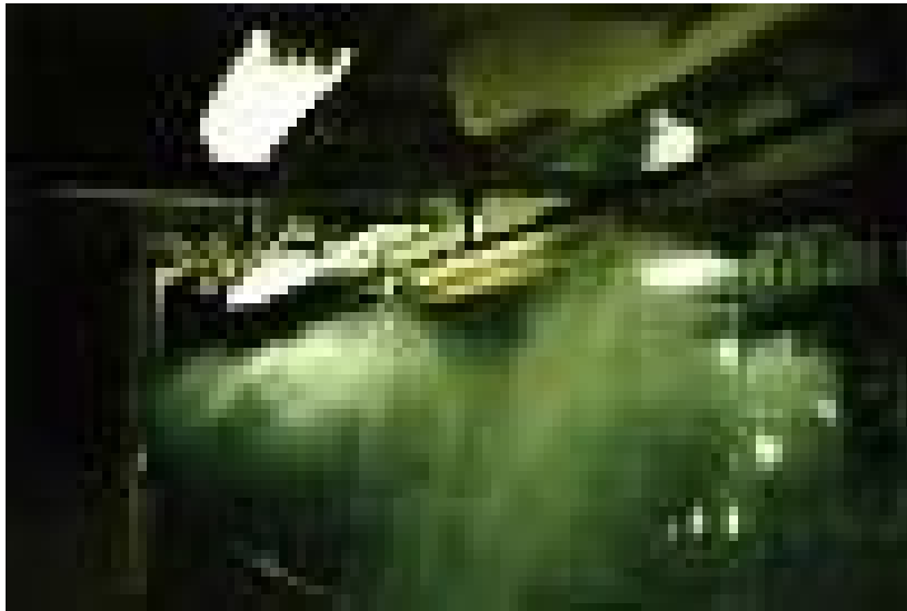
LOW PRESSURE WATERMIST IN MACHINERY SPACE
