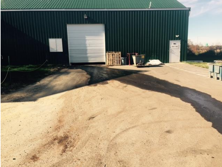
13. Water flowing under the door.
