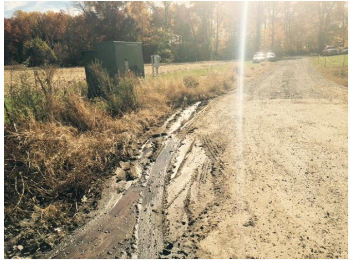
12. Some red material on the ground from the water flowing under the door and the bins.
