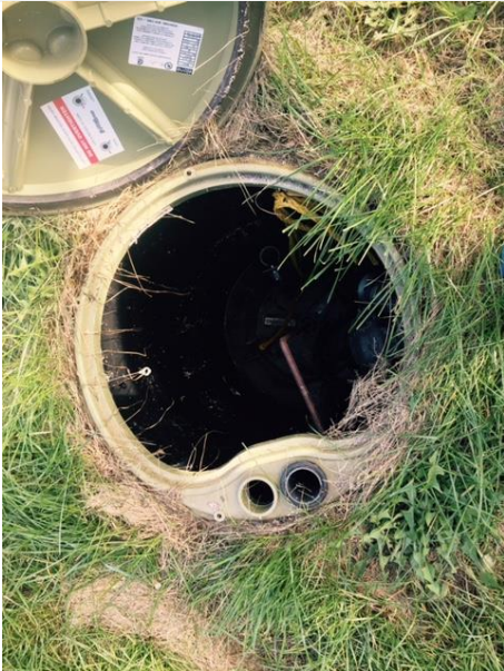
15. The sewer ejector pump.
