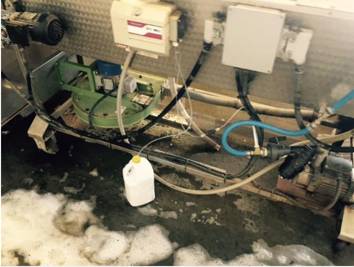
9. The board washer, soap and associated sanitary sewer drain.
