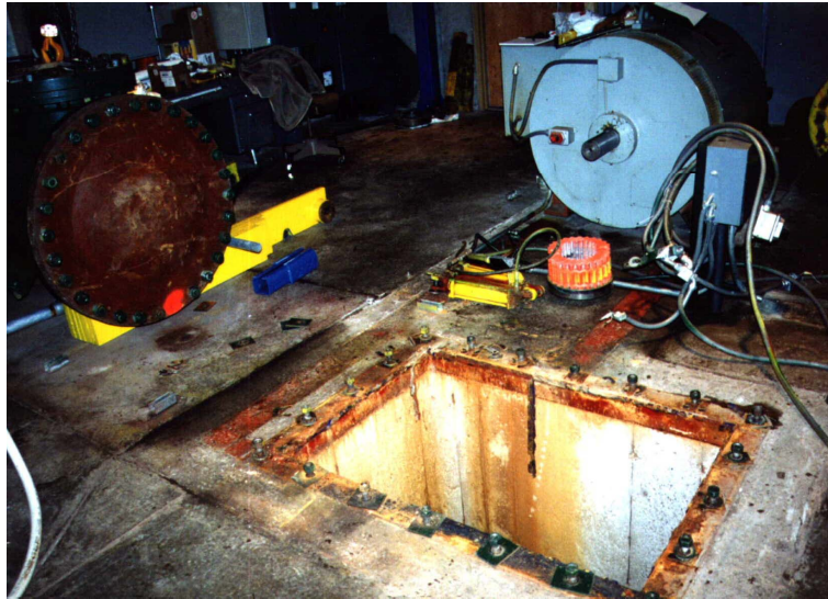
Figure 2: Space for the new Cross-Flow turbine is limited. The water intake flange on the left side, the floor opening for the turbine discharge and the generator shaft in the background. Turbine and gearbox had to fit between.
