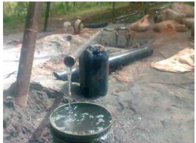
Water running at the new well
