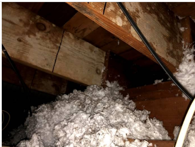
5. Photograph taken looking into attic shows roof/ceiling joists bearing on center load-bearing wall.
