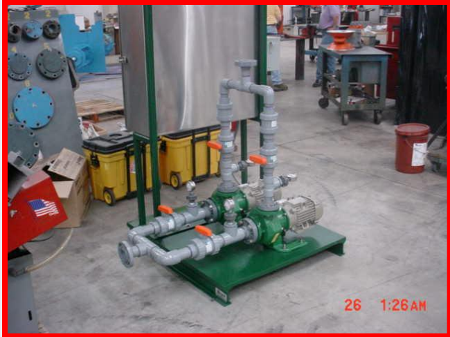
Sodium Hypochlorite Injection system utilizing Non metallic mag-drive pumps.
