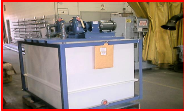
Used for portable chemical injection in wastewater treatment plant.
