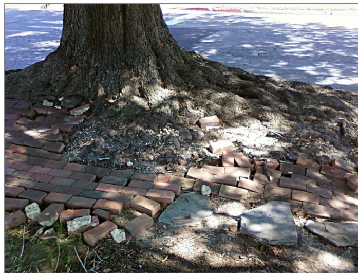
Figure 16: Poor Sidewalk Condition along Americana Drive
