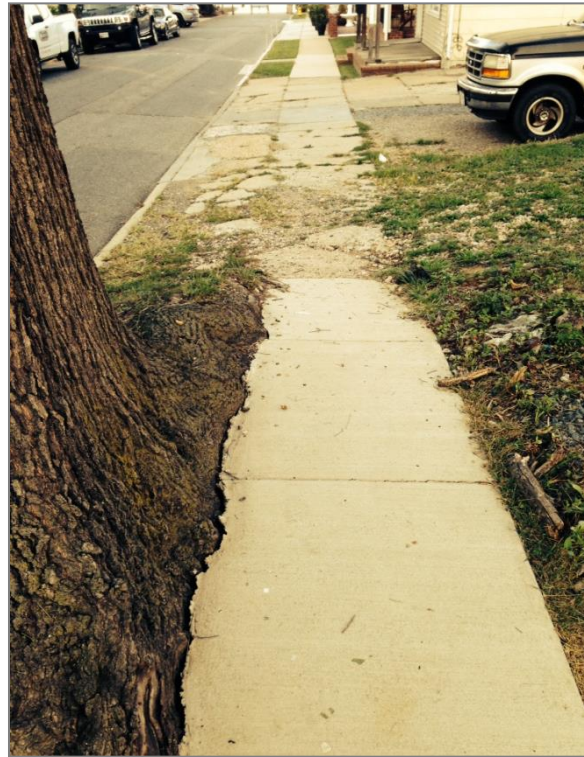
Figure 15: Deteriorating Sidewalk on Severn Ave
