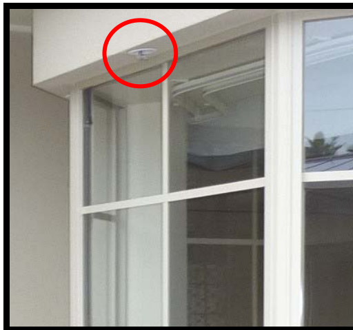
Figure 2 - External Sprinkler Installation
