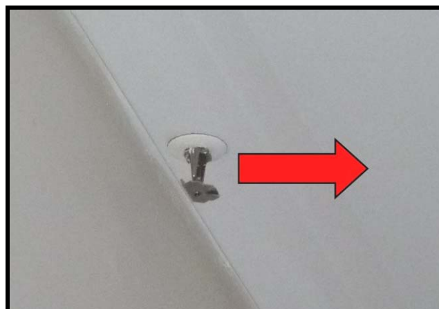
Figure 3 – Sidewall Sprinkler Installation
