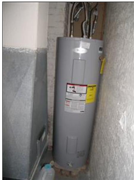
6.7 Picture 1 no containment
