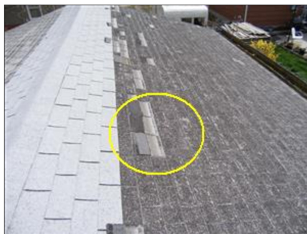
1.0 Picture 4 missing shingles
