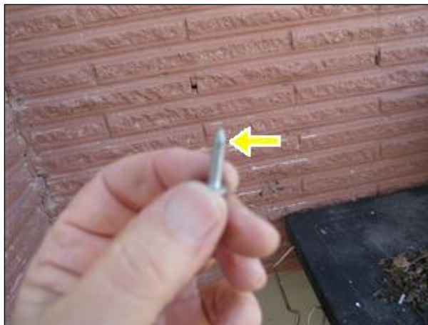
7.2 Picture 3 wrong screws
