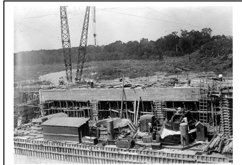
Gunter, Herman, Hydro-electric plant - Jackson Bluff. 1929. Black & white photonegative. State Archives of Florida, Florida Memory. 125104
