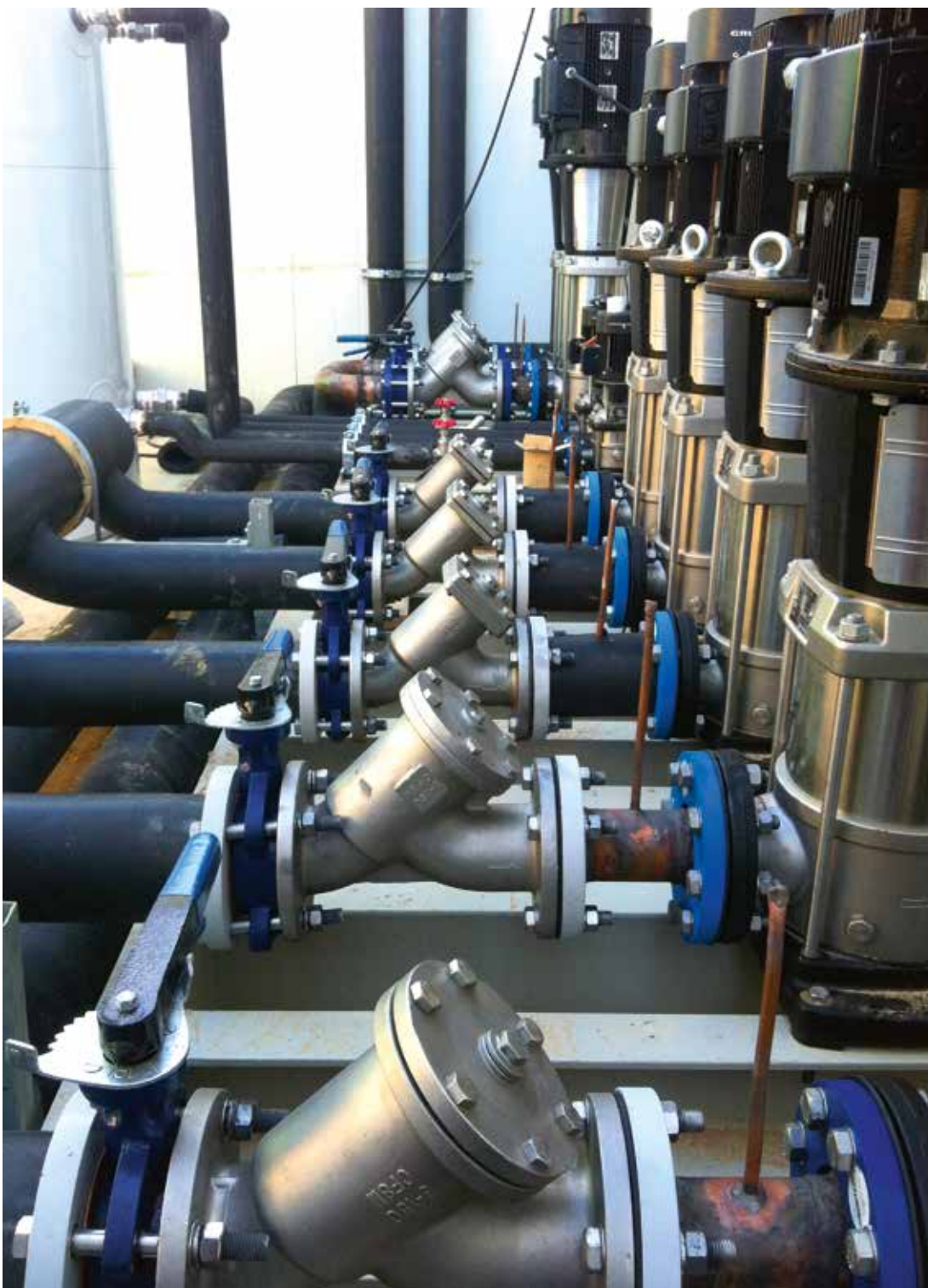
Secondary fluid pumps that circulate HC30.
