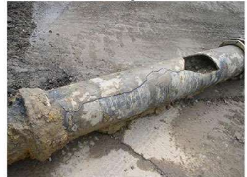
Cast Iron Pipe Broken from Water Hammer
